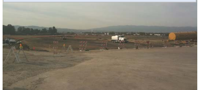
View of future Isabel Avenue looking south towards Interstate 580 from the intersection of future Isabel Avenue and Portola Avenue (11/09)
